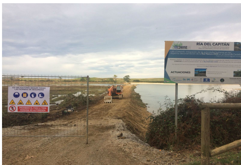
Hydrodynamic restoration project of the marshes in the Ria del Capitan (Cantabria). Source: ConviveLife
