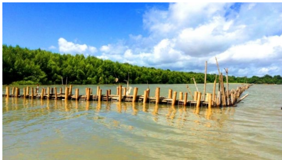
The semi-permeable structures as sediment trap, Sawah Luhur village, Serang-Banten, West Java © Setyawati/MFF-Indonesia, 2016
