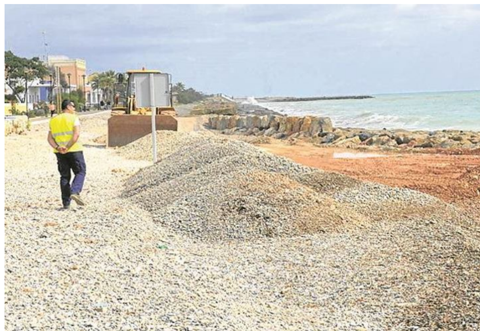
Gravel backfill in Almenara, Spain. Source: Dirección General de Costas, Government of Spain.
